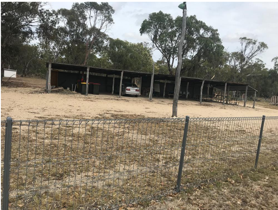
Cement floor open skillion shed. Used for storage for bollards etc for the Sapphire City Motor Sports Club.
