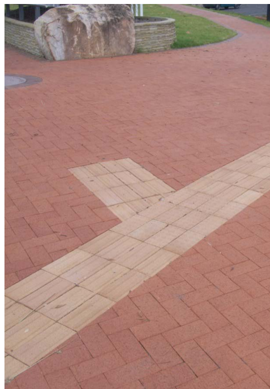
Figure 8 : A typical CBD footpath in Inverell that can require regular inspection due to movement in the pavers causing trip hazards and unevenness
